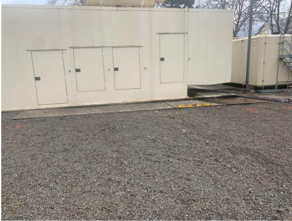
Photo 1—Sidewalk and general ground slope to south in front of existing level generator pad.
