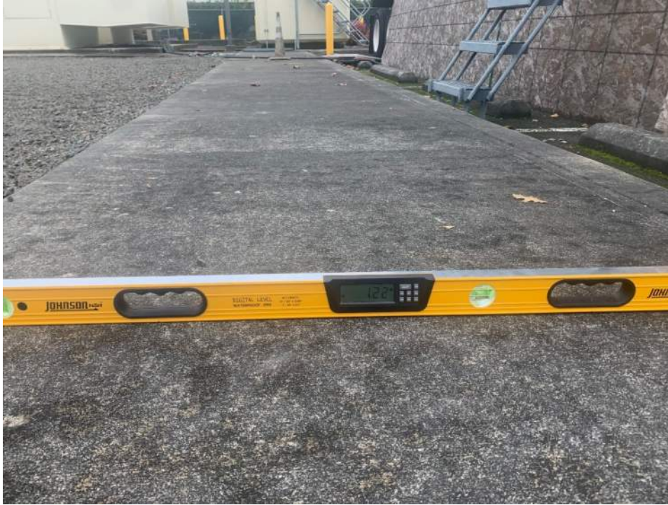
Photo 3—Approx 1.2% slope to south across sidewalk at parking lot.
